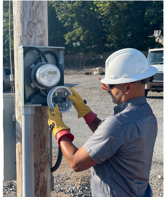
LREC Walter Pigeon, installing meter socket surge protector.
